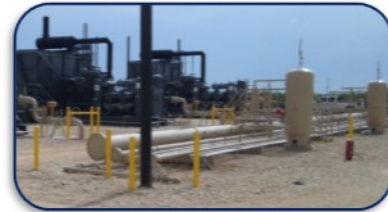
LMS Gas Lift Compressor Station
