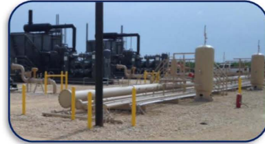
LMS Gas Lift Compressor Station
