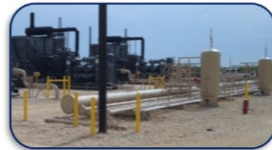
Centralized Natural Gas Compressor
