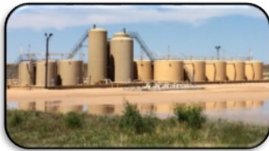
Water Treatment Plant
