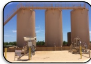
Centralized Crude Gathering Tanks at Reagan Truck Station
